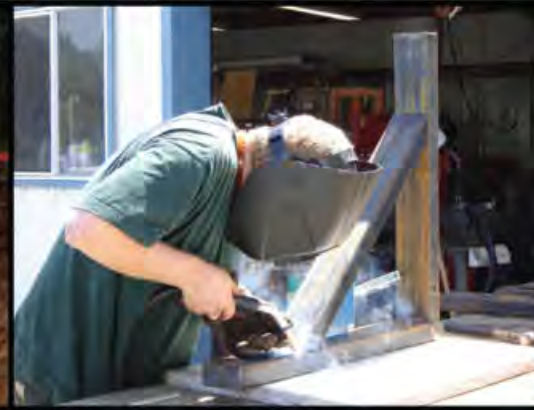
METAL BRACKETS & DINING ROOM CEILING WELDED BY JOHN MOORE, a member of the DC Team
